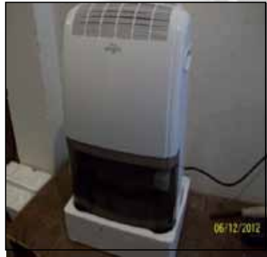
Fig. 47c: Dehumidifier installed inside Breeding Room of Snow Leopard ( Uncia uncia )
