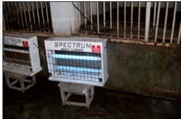
Fig. 24d: Insect Flasher installed inside the night holding pens.
